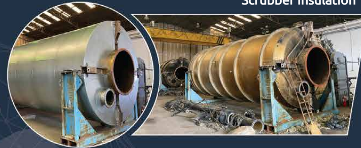
Exhaust Pipes Insulation
